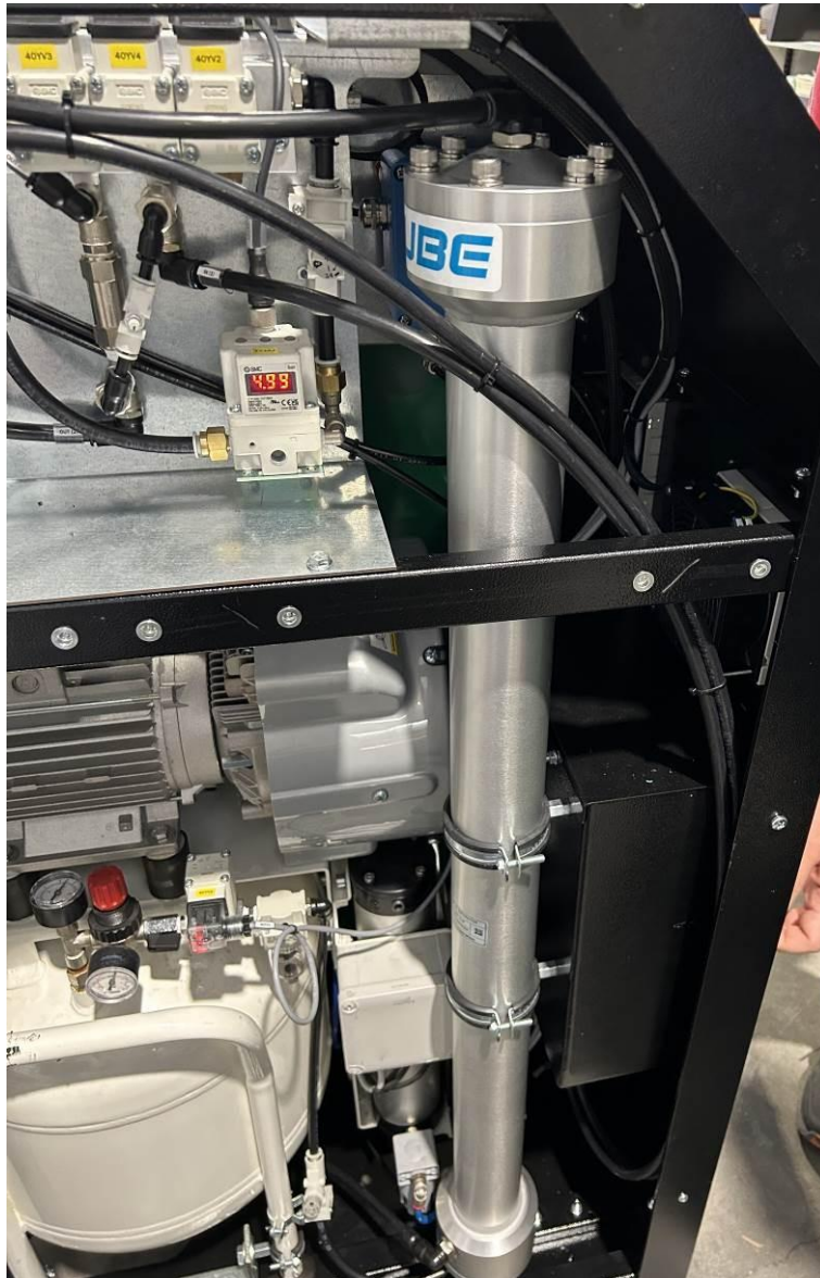
Photo 4.7 – Column filter separator
